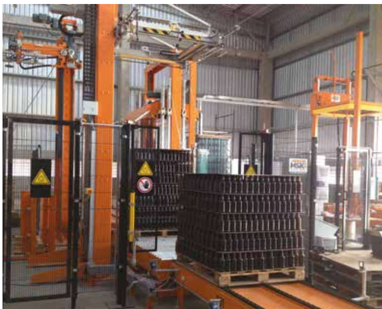
For the third production shop at Vidroporto, MSK delivered the complete cold end from the Lehr exit to pallet packaging.
