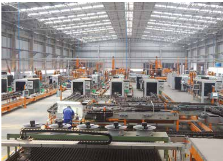
Bucher Emhart Glass FleXinspect inspection machines are installed at the cold end.
