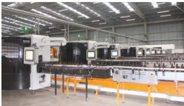
The total number of Bucher Emhart Glass cold end machines in use at Vidroporto now stands at 28.
